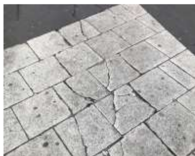
Figur 5. Spruckna plattor (Tyréns, 2020)
