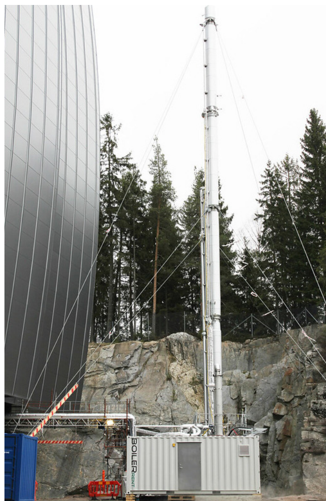
The CO 2 capture pilot plant at the Fortum Oslo Varme plant, showing the absorber and desorber towers. (Photo: Fortum Oslo Varme)
