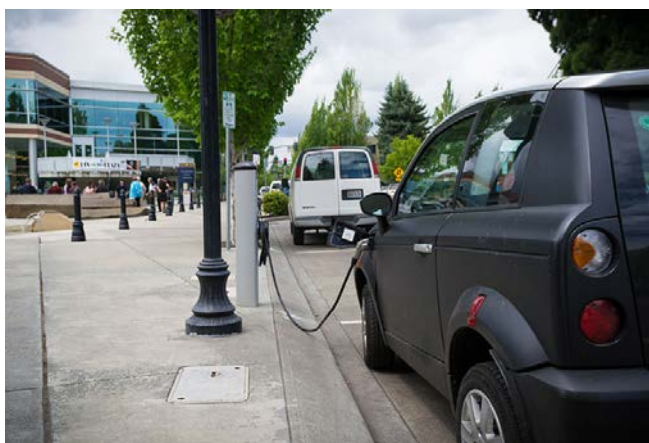
An Electric Vehicle Charging Station (Photo: Wikicommons)
