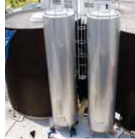
Storage of co-substrates in arabern plant
