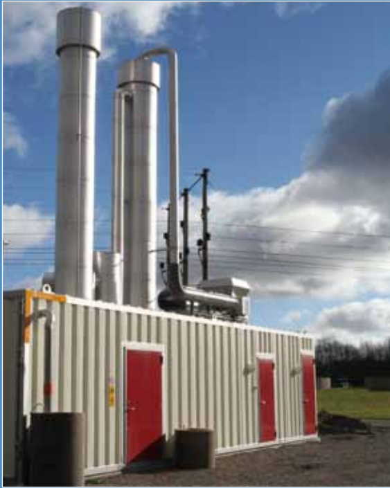
Upgrading unit in Falköping
