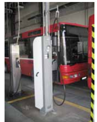
Indoor filling station
