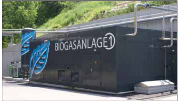
Gas upgrading plant (PSA)
